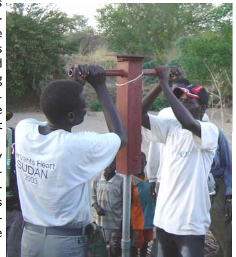
Country Manager Deng Leek works with his assistant to dig another well in Daga Post. Servant’s Heart is working to bring clean water to ten villages in 2005. River water is full of silt and water-borne disease.
